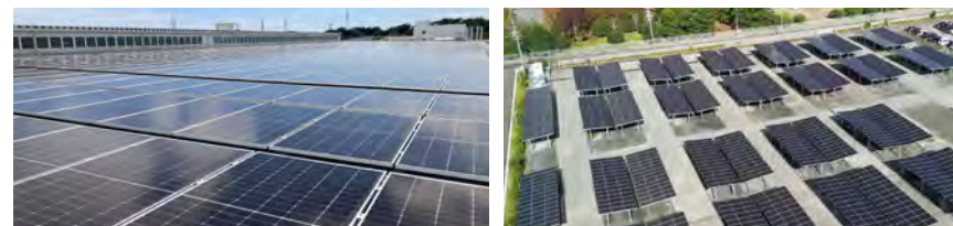
Solar panels installed at the Kakegawa Factory
