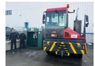
Bio-Fuel Station (Unipres (UK))
