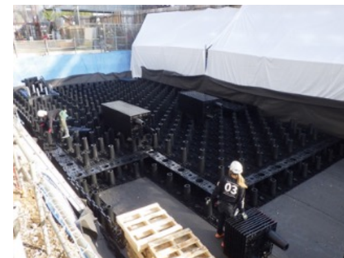
Underground Rainwater Retention and Infiltration Tank
