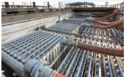
Image of a wastewater reclamation system installed at a customer's plant
