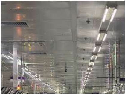
Switching to LED lighting in the factory
