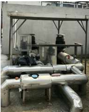
Pure water production system
